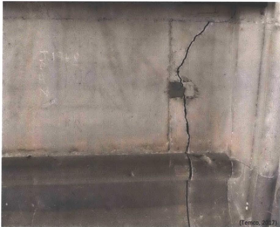
Figure 7: Cracked stone at Winchester Cathedral
