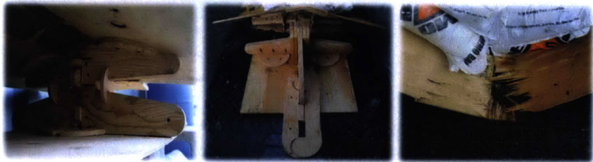
Fig. 5.24 Failure Modes – GEN.3_Semi-unitized: (a.) Pedestal; (b.) Lower Flange; (c.) Upper Flange.
