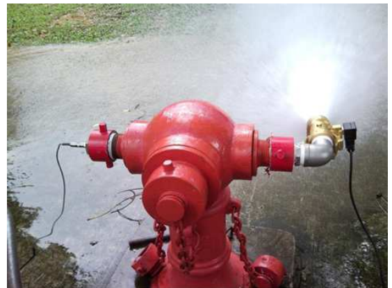
Fig. 13. Fire Hydrant that is used to create simulated bursts during the leak-off experiment
