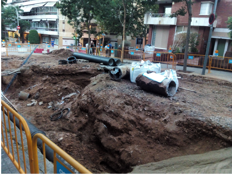
Figure 1-1: Carrer Ganduxer, Barcelona, after water mains burst[7]
