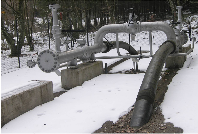
Figure 1-2: A crossover station to allow for temporary flow stoppage and pig insertion[9]
