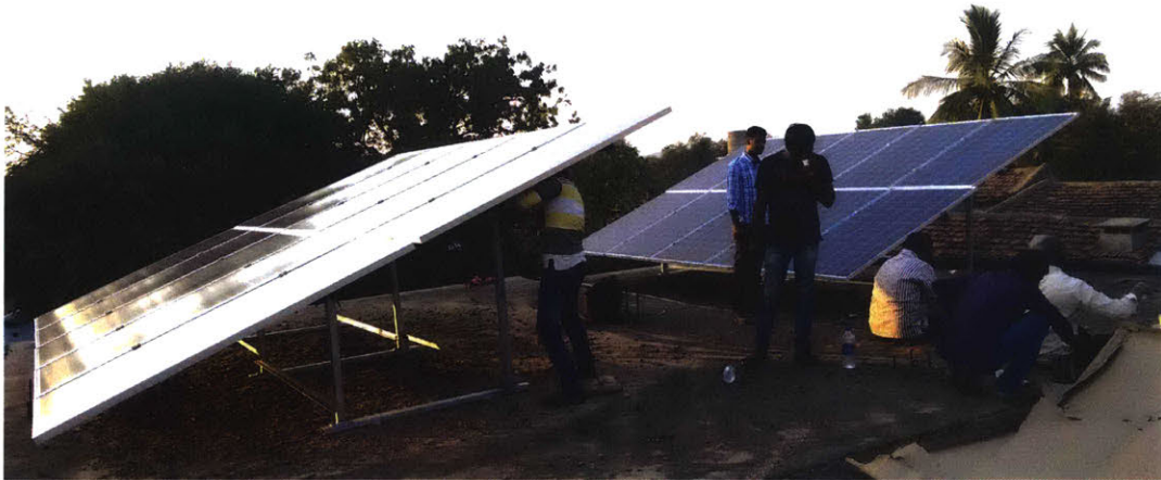
Figure 4-2: Actual solar panels installed on the rooftop of the building housing the desalination system in Chelluru.
