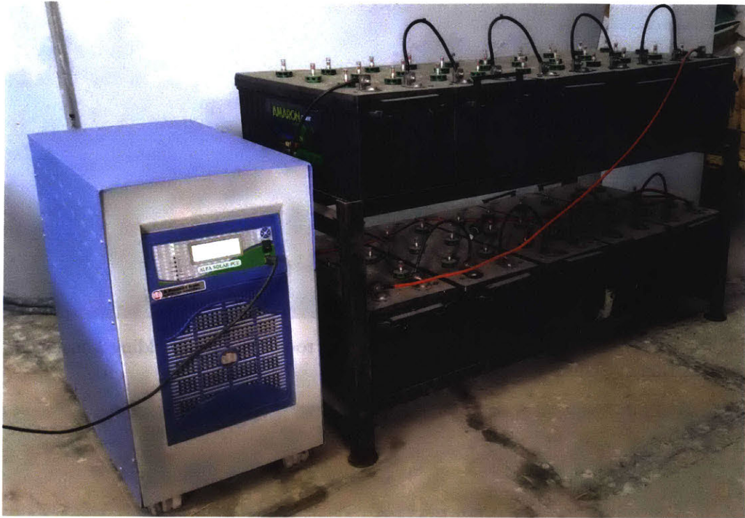
Figure 4-4: Actual inverter (left) and batteries installed in Chelluru.
