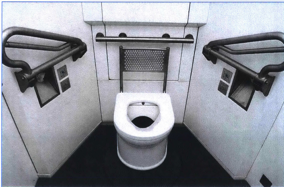
Figure 3: Automatic Public Toilet, Boston
