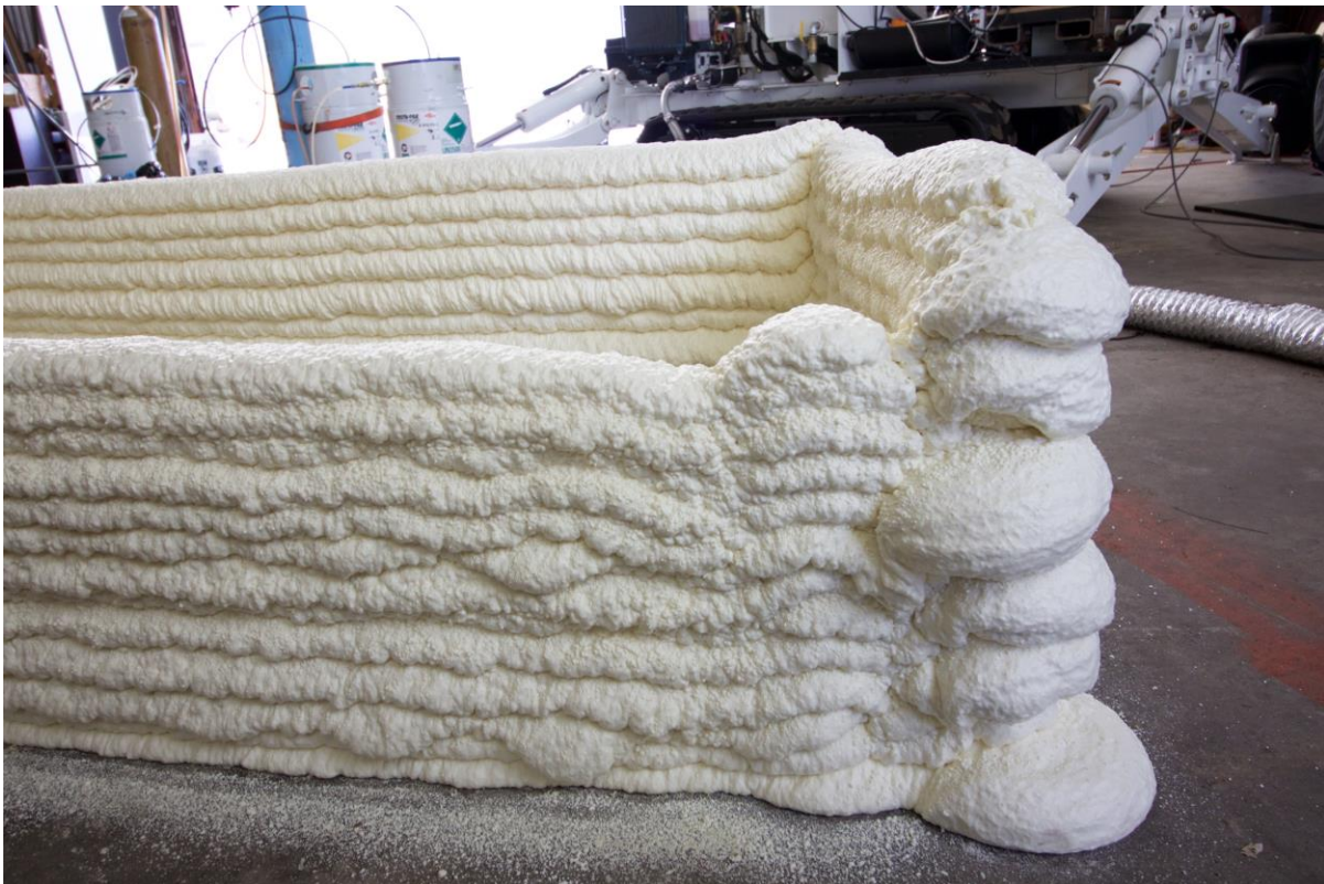
Figure 35: Foam build-up at corner of curved wall section. Image credit: Steven Keating.
