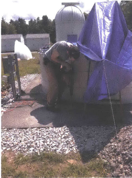
(i) 22 July 2014 - Tim Brothers drilling into the concrete pad to attach the base ring.
