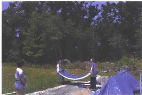
(g) 22 July 2014 - Megan Russel, Rachel Aviles, and I constructing the dome ring.
