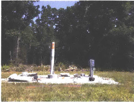
(a) 24 June 2014 - Cutting the four foot concrete pier to six inches above the concrete pad.
