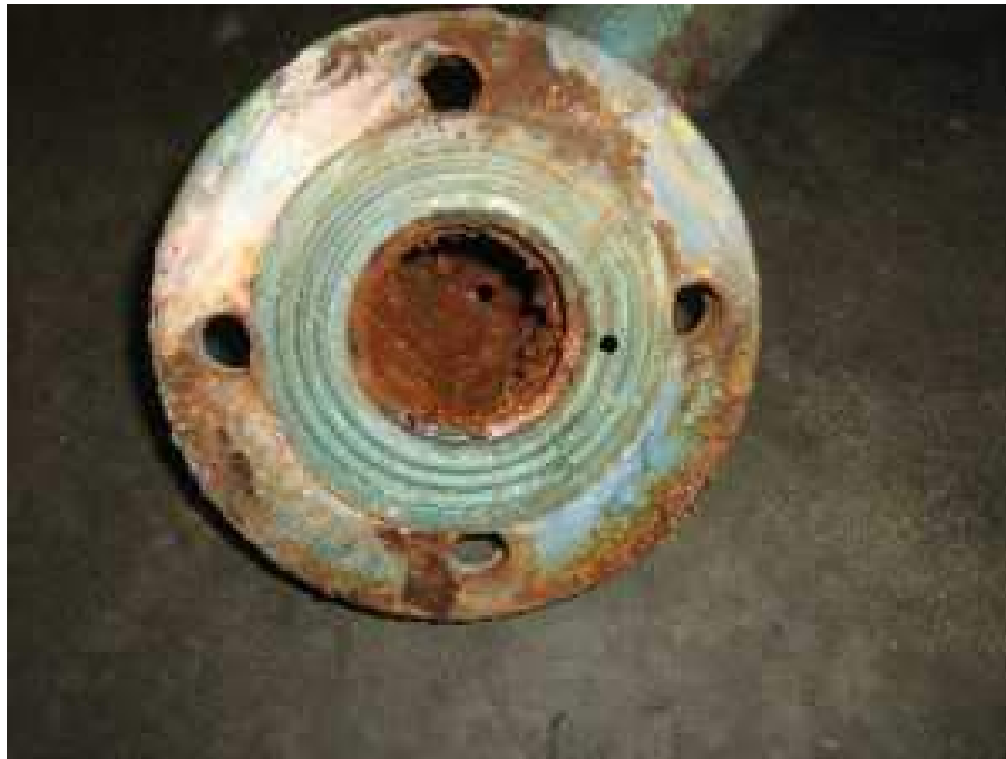
Figure 2-5: This figure shows a corrosion fouling of steel within a cooling water pipe of an industrial heat exchanger of the Nuplas Industries plant [63].
