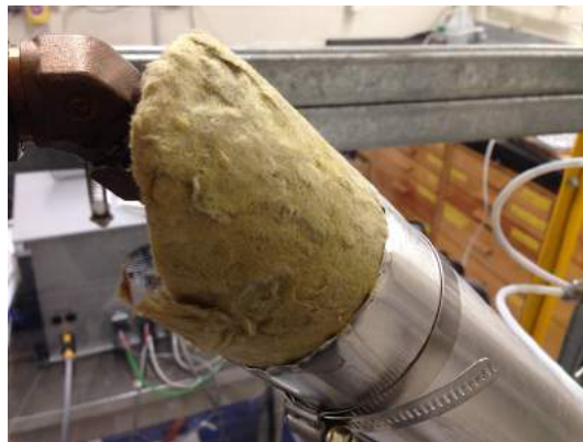
Figure 3-59: Ceramic wool heat insulator. Yellow ceramic wool is covered by its aluminum sheet jacket.
