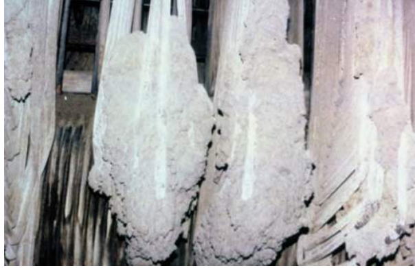
Figure 2-2: This image shows ash fouling deposits on superheater tubes in a coal-fired power station [14].
