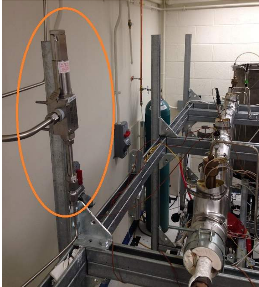
Figure 3-53: Photo of main loop RVP pressure relief valve.
