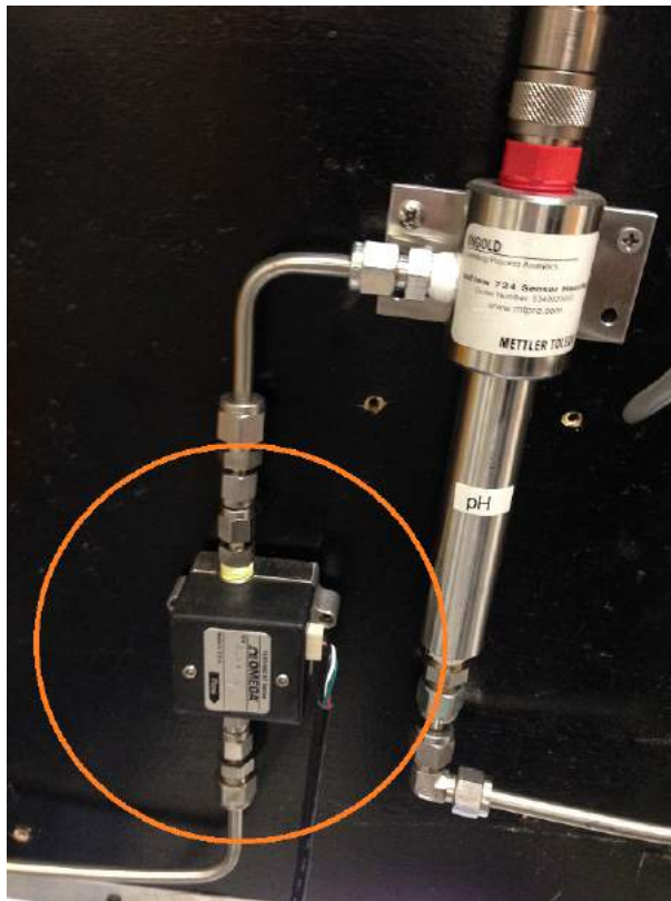
Figure 3-69: Photo of auxiliary loop flow sensor.
