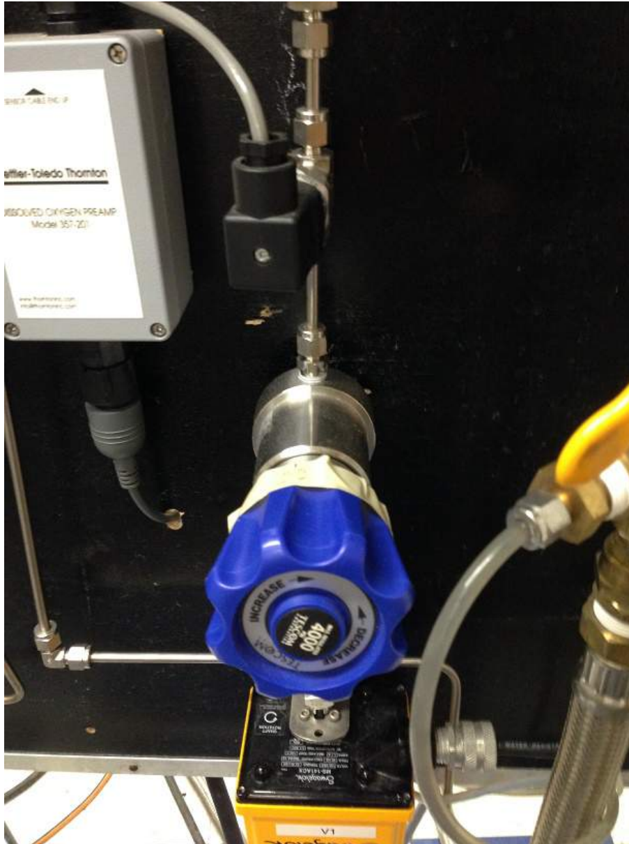
Figure 3-74: Photo of back pressure regulator.
