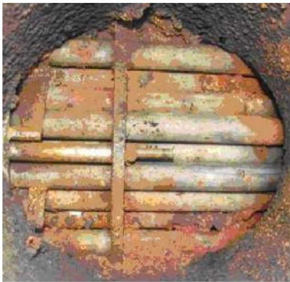
Figure 1-3: This image shows an example of corrosion fouling, in the form of red rust produced by the corrosion of low-alloy steel with surrounding water. The fouling material results from the reaction between the process fluid and heat transfer surface [16].
