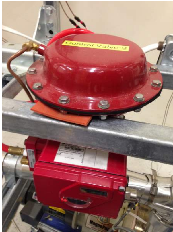
Figure 3-18: Photo of IHTFP's control valve 2.
