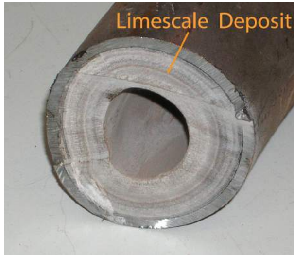
Figure 1-4: This figure shows a limescale layer in a heat exchanger pipe. Its thickness reduces the area through which the fluid can flow, and deteriorates the heat exchanging capacity of the pipe [21].
