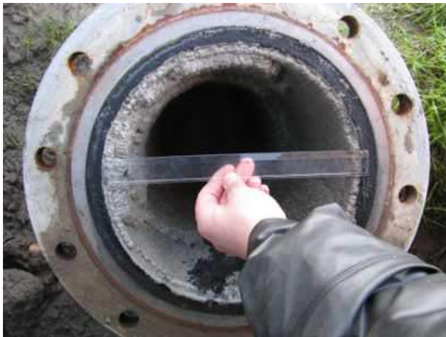
Figure 2-6: This image shows a thick limescale layer in an oil refinery effluent pipe. The thick layer in the pipe is the limescale layer [64].
