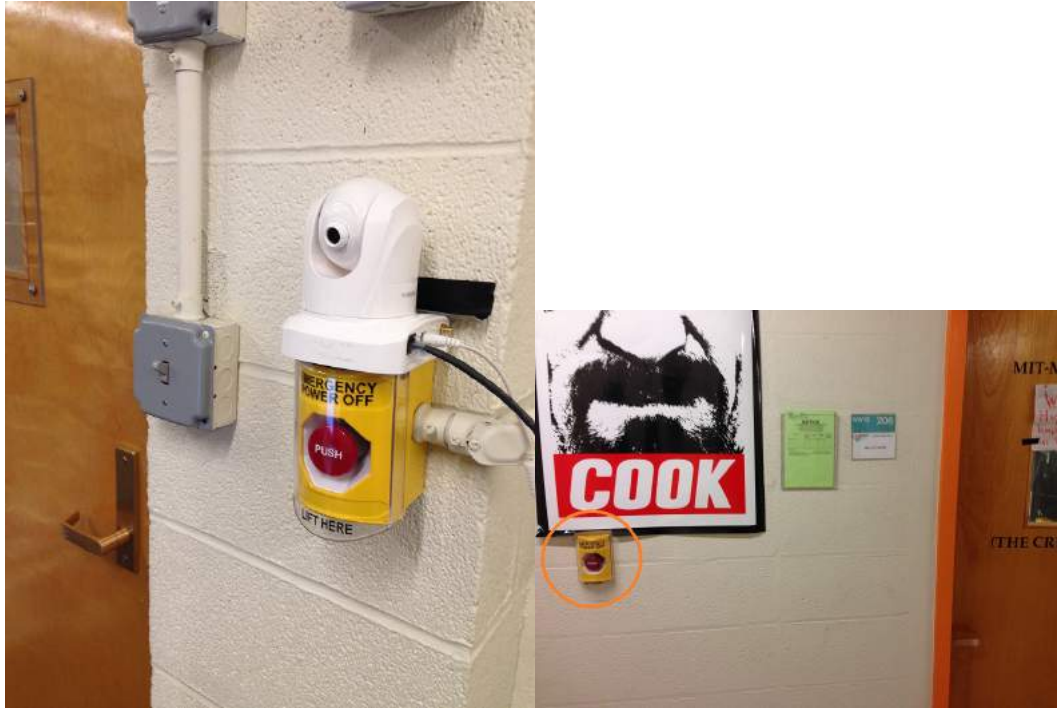
Figure 3-42: Photo of emergency switches inside the room (left) and outside the room (right). These switches will close down all power including that of pressurizing pump. They should only be used as last resorts.
