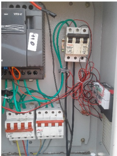
Figure 5: Solar Pump System Electronics (detail)
