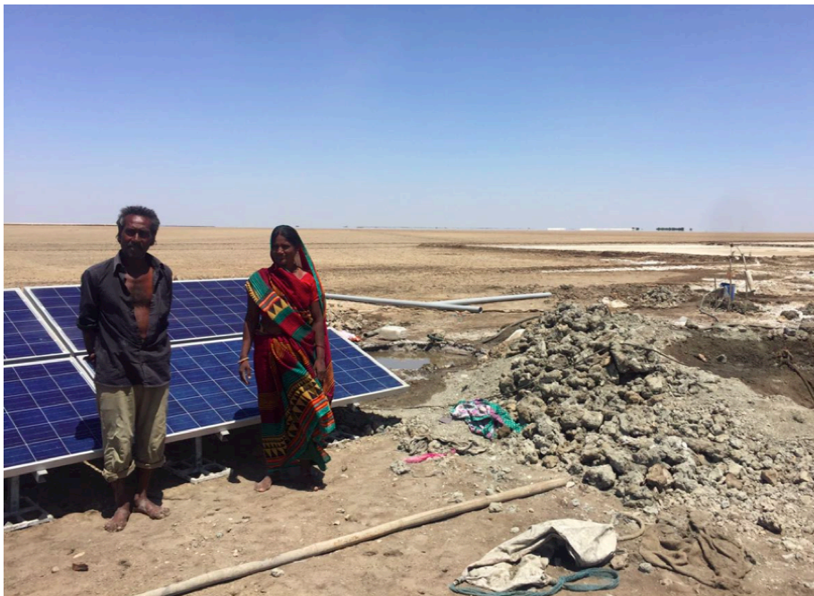
Figure 10. Solar Pumping for Salt Production in Gujarat
