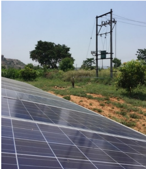
Figure 9. Grid-Powered Solar Pumping in Karnataka
