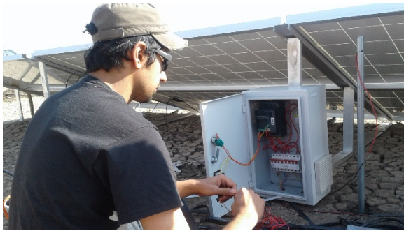
Figure 4: Solar Pump System Electronics
