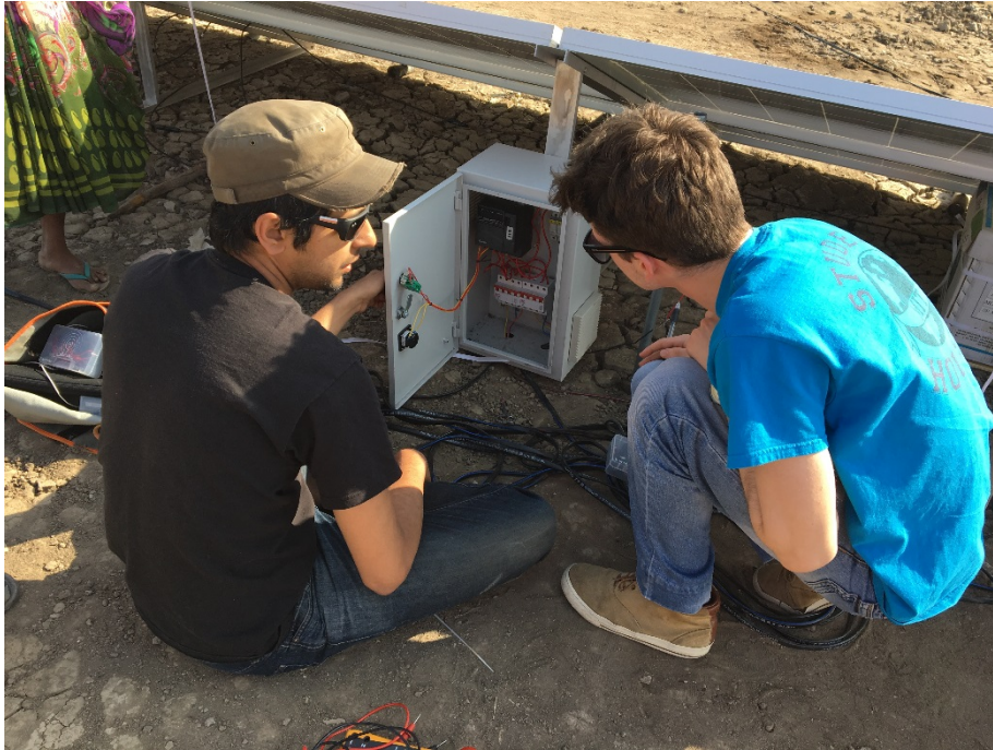
Figure 50: CITE Researchers Amit Gandhi (left) and Przemyslaw Pasich (right) Installing Sensors
