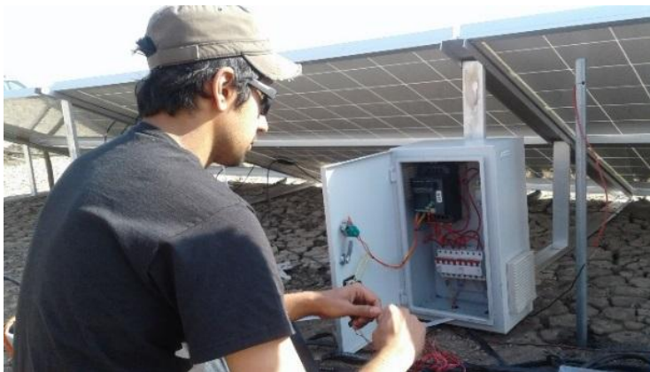
Figure 3: Solar Pump System Electronics
