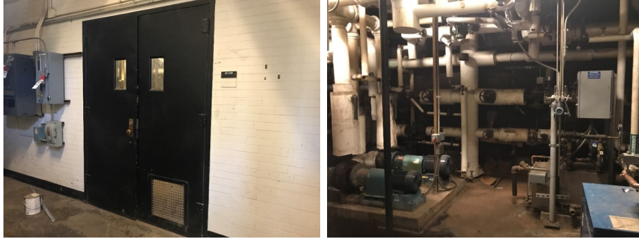
Figure 4-6: Photographs of exterior and interior of the machine room in the basement.
