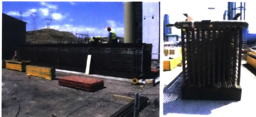
Figure 4-3. Photo of HTF tubes imbedded in concrete storage system at DLR 161
