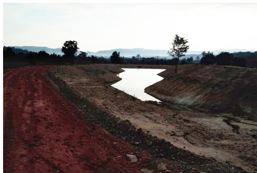
Exhibit 3-12: Yoob-Hua-Chang dam | photographed and written by Sarawut Nakun (Wut) for the end-of-workshop photo exhibition
