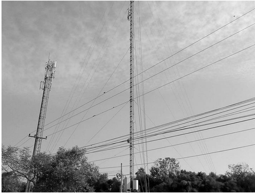
Exhibit 2-7: Cellular Towers | photographed by Pornjarat Tunpirat (Un)
