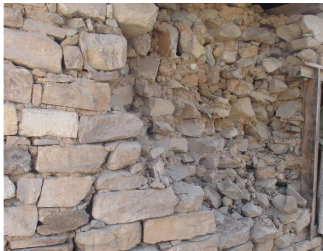
Figure 94: Out of plane failure of mud and stone wall (Chitlang, Nepal)
