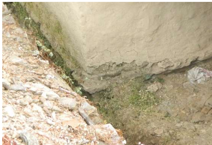
Figure 16: Conventional mud-based exterior plasterwork in Chagam, Nepal showing cracking and sloughing
