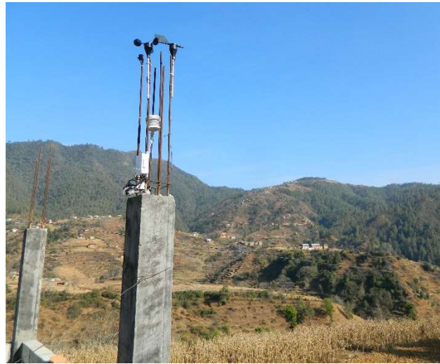
Figure 85: Onset Computer Corp. HOBO H21-002 weather station installed in Chitlang, Nepal
