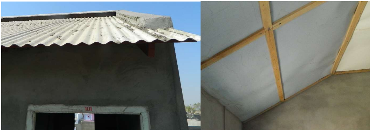
Figure 67: Corrugated Metal Sheet roof with Bubble Wrap and Metal Sheet roof section (Nelson, 2017) and as-built
