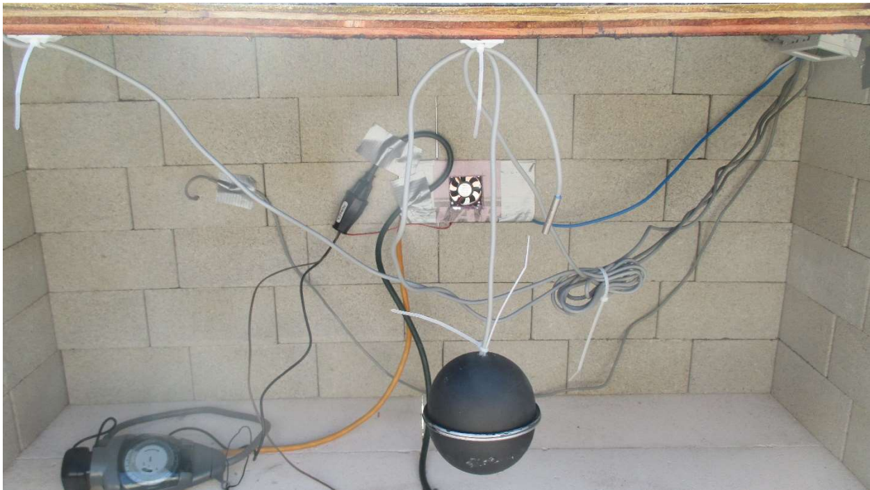
Figure 4: Metering and electrical components of testing chamber, prior to wire routing
