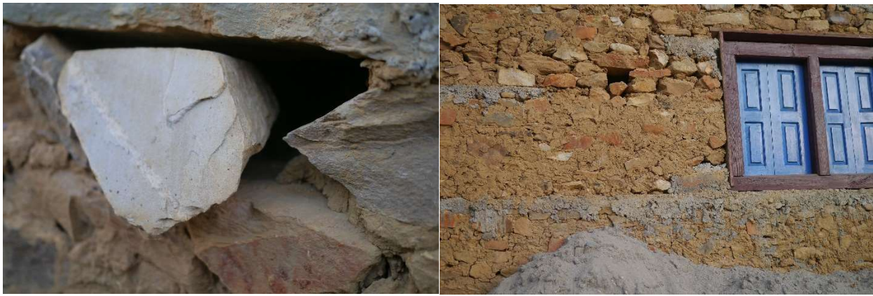
Figure 93: Loose and missing stones in a typical home construction, showing baseball sized cavities. (Chitlang, Nepal)
