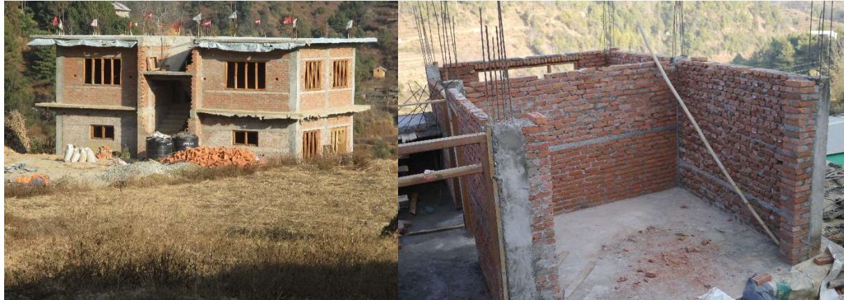
Figure 83: Active RCC Construction projects (Chitlang, Nepal). Left: Builder constructed, Right: Owner constructed
