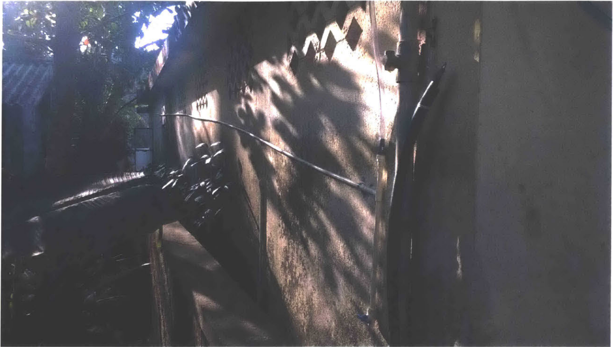
Figure 7: Piping for the gas
