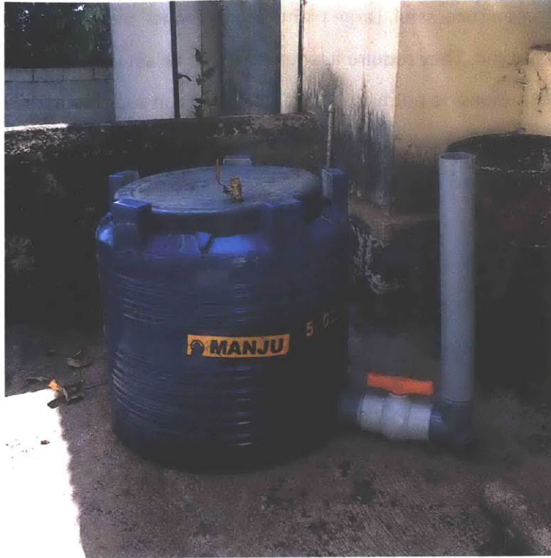
Figure 12: A 0.5 m 3 plant at a small household
