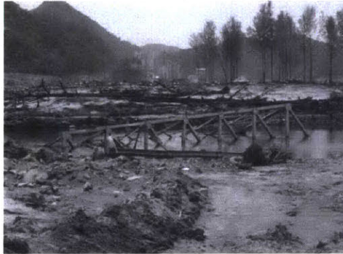
Figure 3- Failure of steel truss bridge by Sumatra Earthquake and Tsunami in Indonesia 2004 [2]
