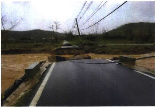
Figure 1- Bridge failure by Hurricane Maria in Puerto Rico 2017, leaves communities without means of evacuation and means of communication for relief efforts [6]
