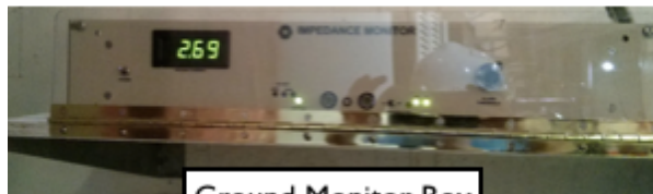
Ground Monitor Box
