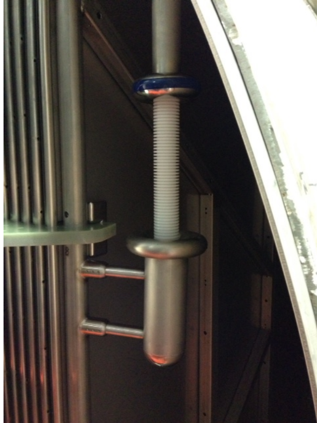
Figure 25. The production HV feedthrough inserted into the cathode receptacle cup inside the cryostat.
