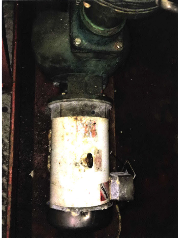
Figure 2-29: Bilge and emergency ballast pump on USCGC SPENCER
