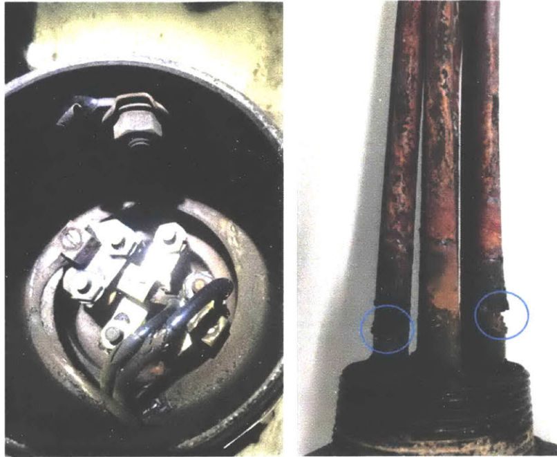
Figure 1-8: Left: Bare wiring found in SPENCER jacket water heater. Right: Holes (circled) in the heating element that allowed water to enter electrical enclosure.
