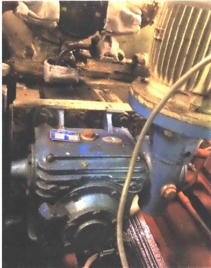
Figure 2-33: Shaft turning gear motor on USCGC SENECA.
