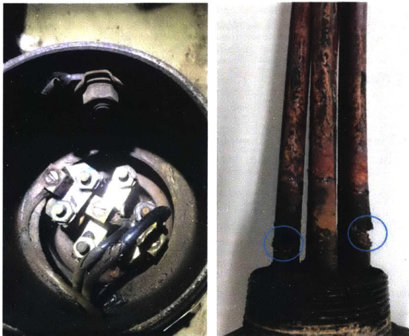
Figure 4-7: Left: Bare wiring found in SPENCER port inboard jacket water heater. Right: Holes (circled) in the heating element that allowed water to enter electrical enclosure.
