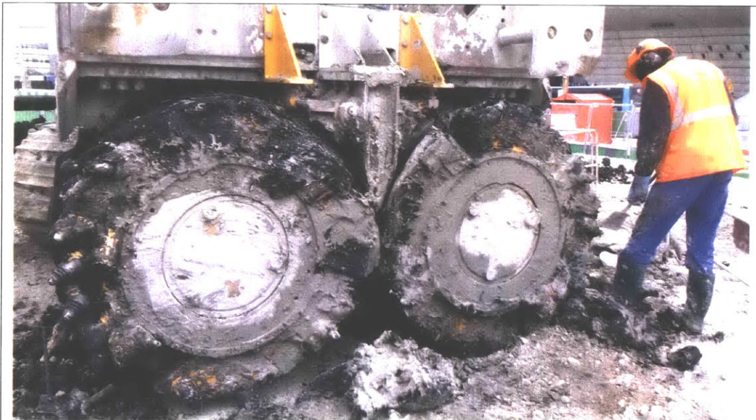
Figure 4. Clogging on the cutter trench of a hydromill in Porte Maillot, Paris
