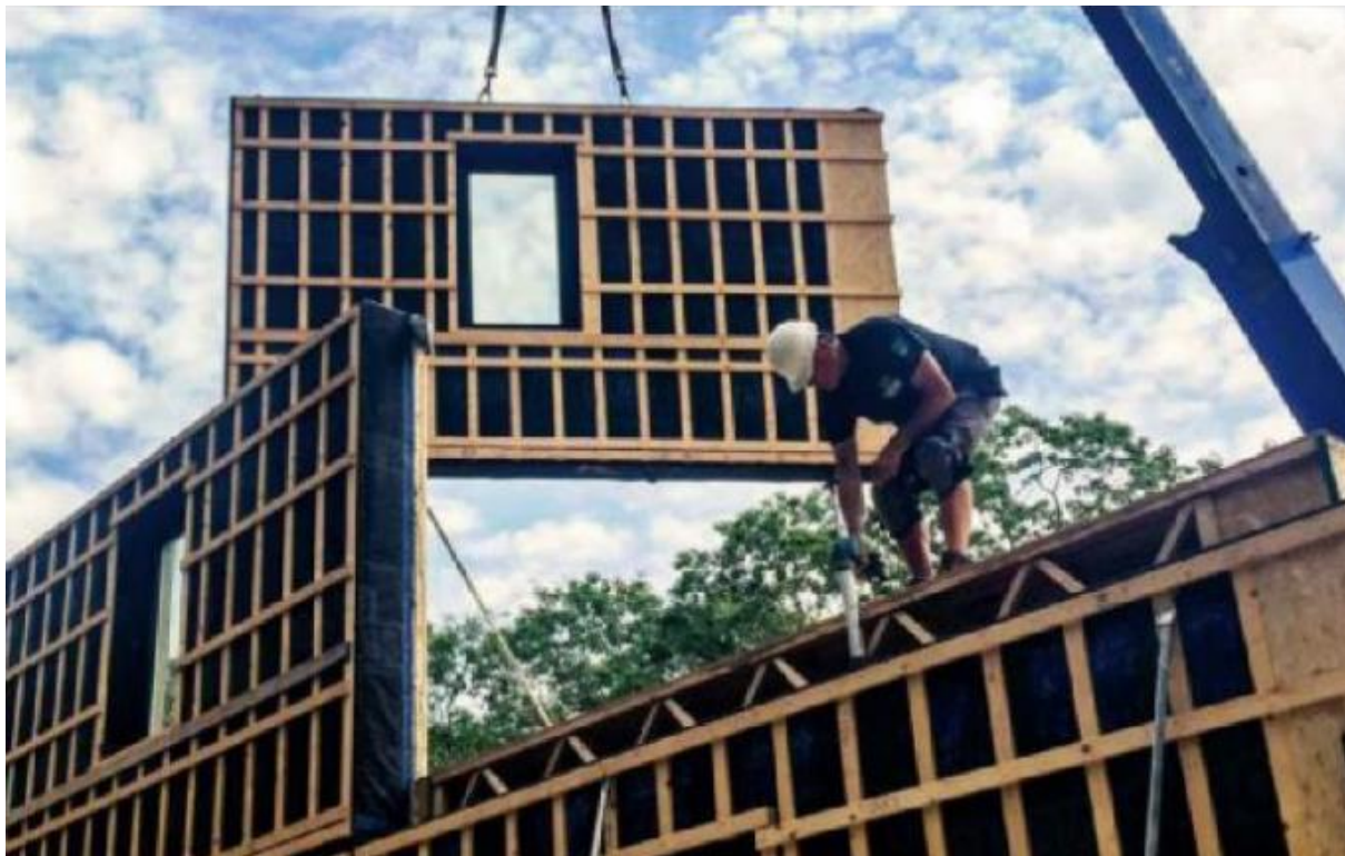
Fig.10: Panelized Standard Walls for island homes in Maine – Construction and assembly as panels. (Data Source: Retrieved from Ecocor official website)
