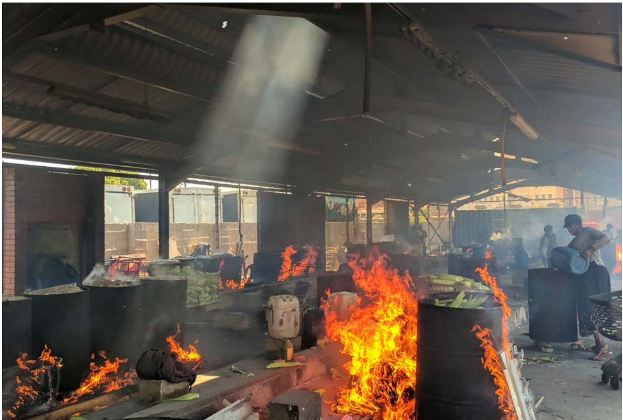
Figure 3.5: Mealie facility after a few months of operation - the result of a bad design process (source: author’s own photo)
