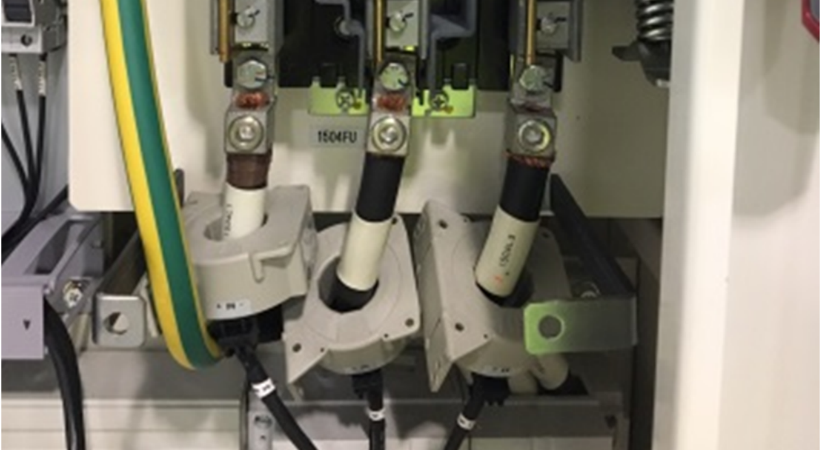
Figure 2-2: A photo of three HARTING Hall effect current sensors installed around three cables. The installation of these sensors required an almost full-day shutdown of the electrical system pictured. A single 200 A HARTING Hall effect sensor can cost $90. Photo courtesy of HARTING corporation.
