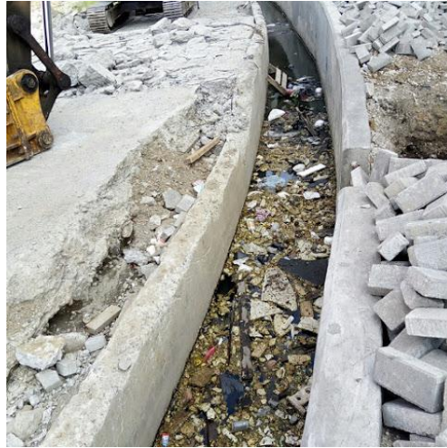
(b) Drain in need of cleaning
