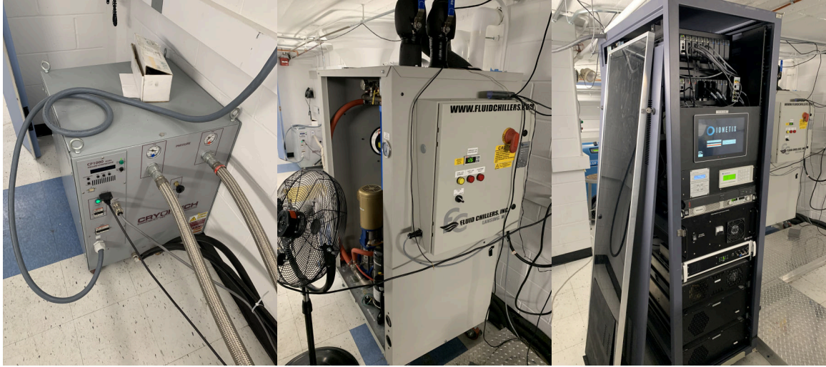
Figure 4-2: Photos of the three main auxiliary components. From left to right is the CPA1110 cryo compressor, WAT 5000 chiller, and the PLC control rack.
