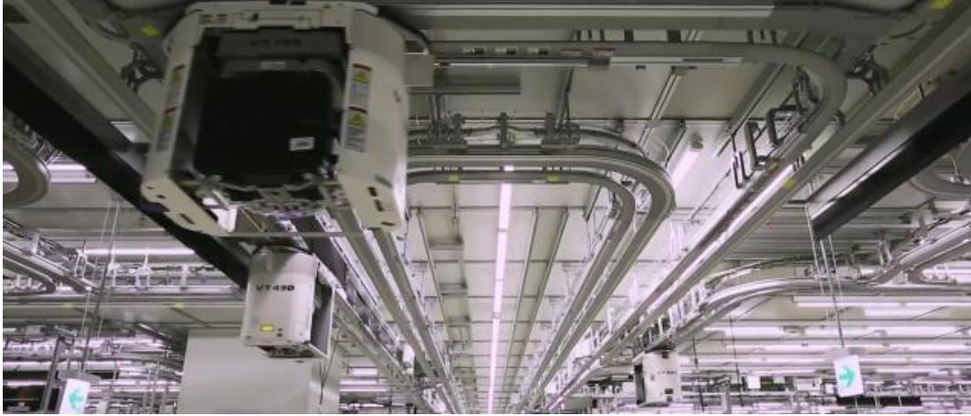
Figure 1-1: A vehicle traveling along the OHT system of a Fab. Image courtesy of Samsung.
