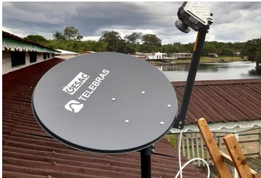
Figure 12. Photo of a satellite dish installed in a school in the city of Monte Alegre, in the Brazilian northern state of Para. (Source: Prefeitura Municipal de Monte Alegre)
