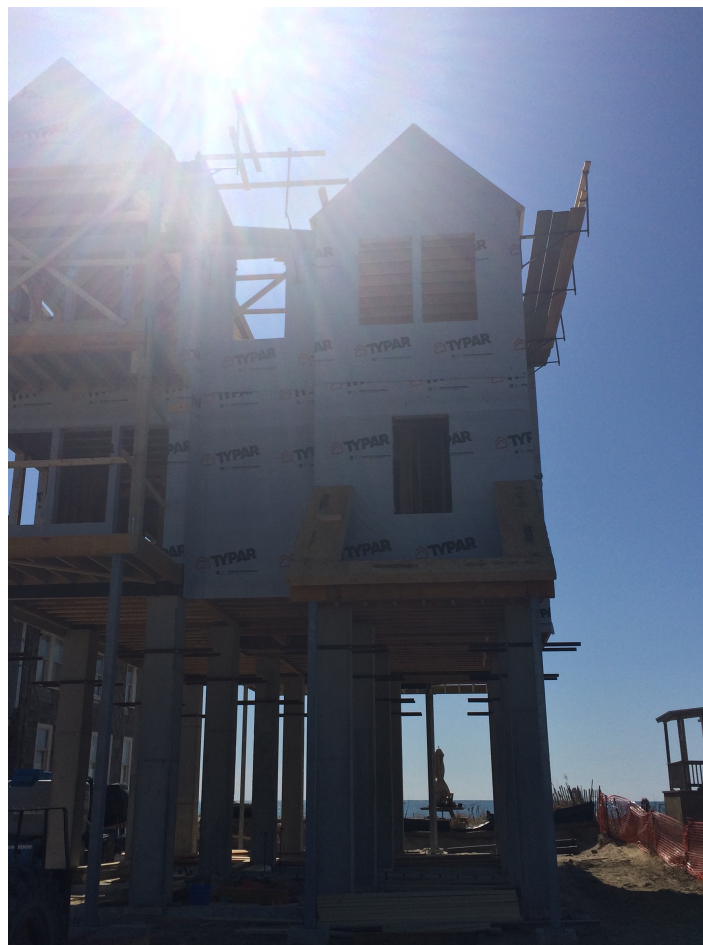
Figure 9: Foundation elevation in progress for a home in East Beach. Source: Regional planning official, 2020.
