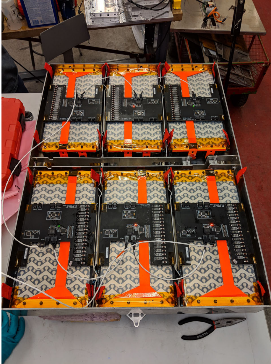
Figure 3-1: Top view of the MY19 battery pack, showing six battery modules connected in series to form the larger pack.
