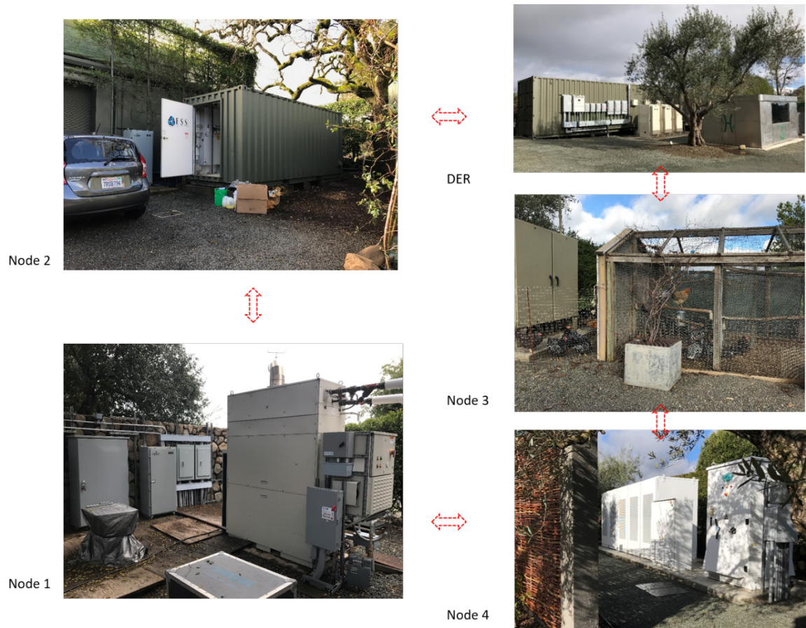
Figure 5-1: Micro-Grid Site at Stone Edge Farm, Sonoma, Cali., Overview of Each Node Described Above.
