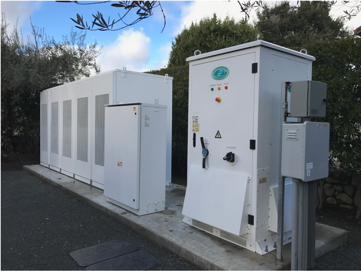
Figure 5-6: Tesla's Batteries and Power Converter System.
