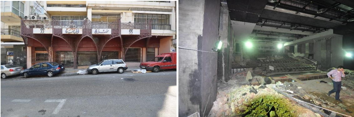
Fig. 41. (Left) Street View of the Space of Saleh Barakat Gallery Before Renovation. Courtesy of LEFT Architects.
