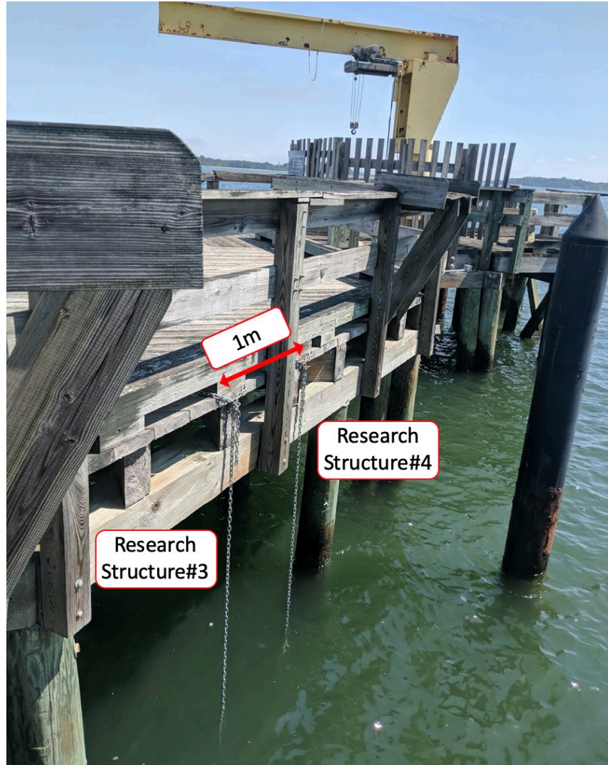
Figure 3.4: South-facing side of Fallon Pier with Research Structure #3 and #4 hung from wooden railing posts with 1 m distance in between.
