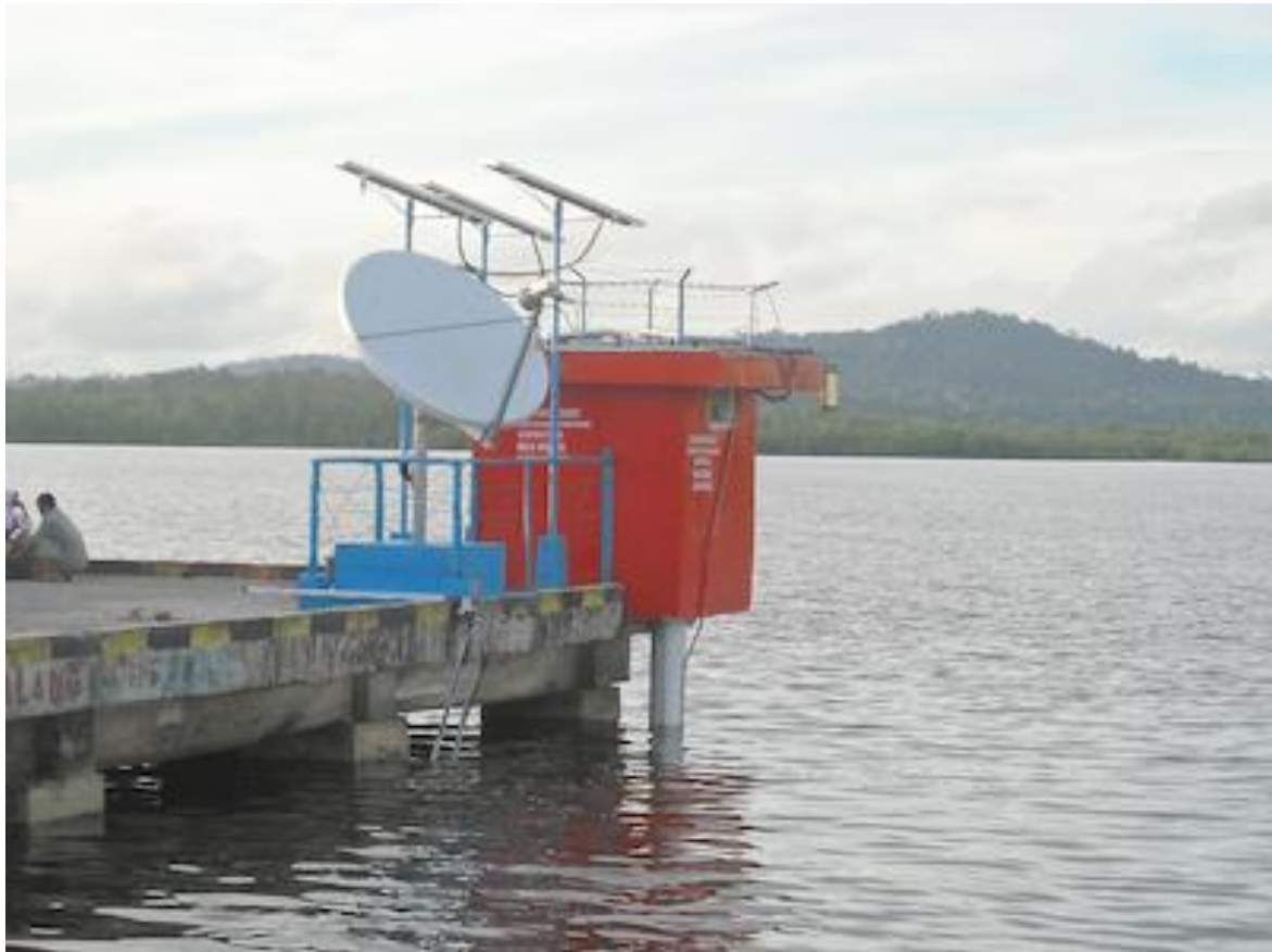
Figure 3-8: BIG's typical tide gauge station with a C-Band VSAT antenna, solar panels and radar gauge hanging by the roof [151]
