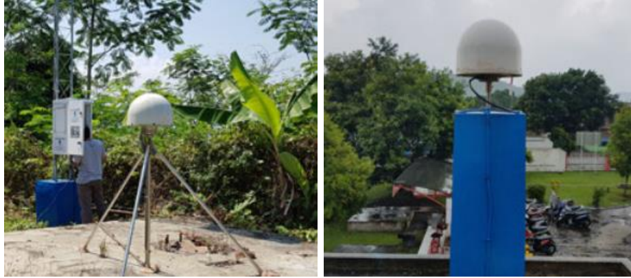
Figure 3-9: BIG's GNSS reference stations [152]
