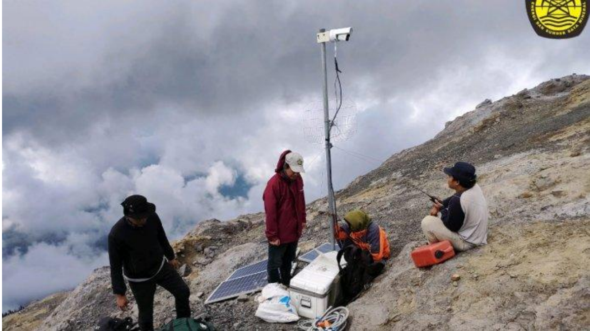
Figure 3-6: A wireless CCTV operated by PVMBG under maintenance [149]
