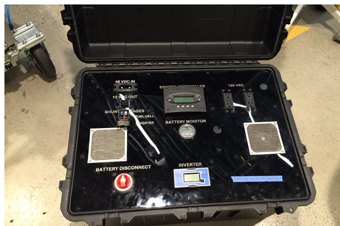
FIGURE 8. Power conditioning components, as well as the batteries and battery management subsystem are housed in separate rugged container for the 3 kW power supply.
