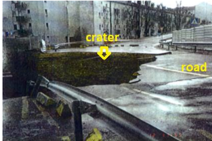
Figure 34 Collapse that occurred in Olivais Station, Lisbon, Portugal (adapted from Appleton, 1998)
