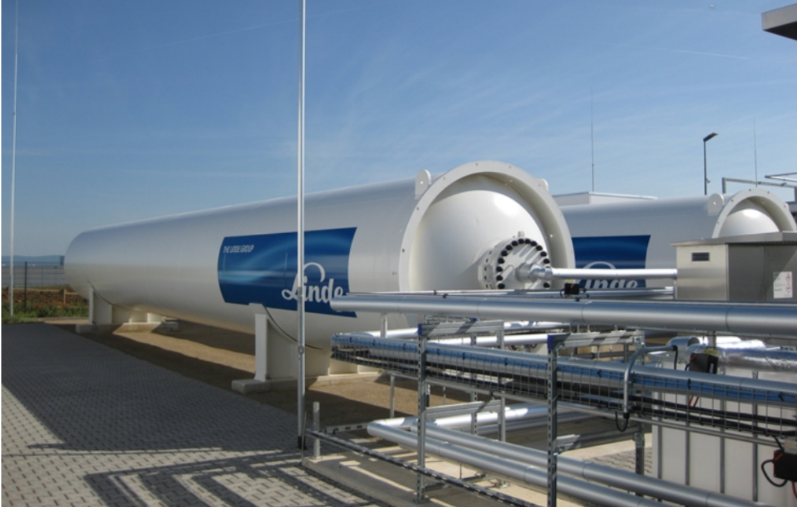
Figure 2-2: Photo of Pressurized Hydrogen Storage Tank [56]
