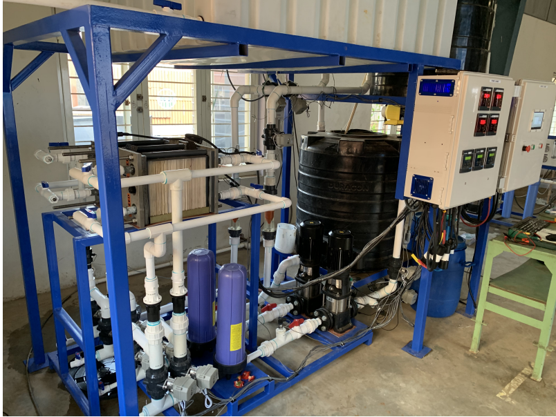
Figure 1-5: Batch ED pilot deployed in Medchal, India. The GEAR Lab collaborated with Tata Projects Ltd. to pilot a 500 L/h ED groundwater desalination system and evaluate its performance against a RO system.
