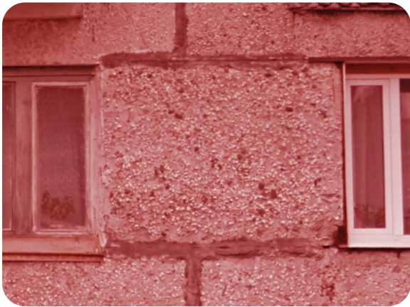
Deteriorating facade joints
