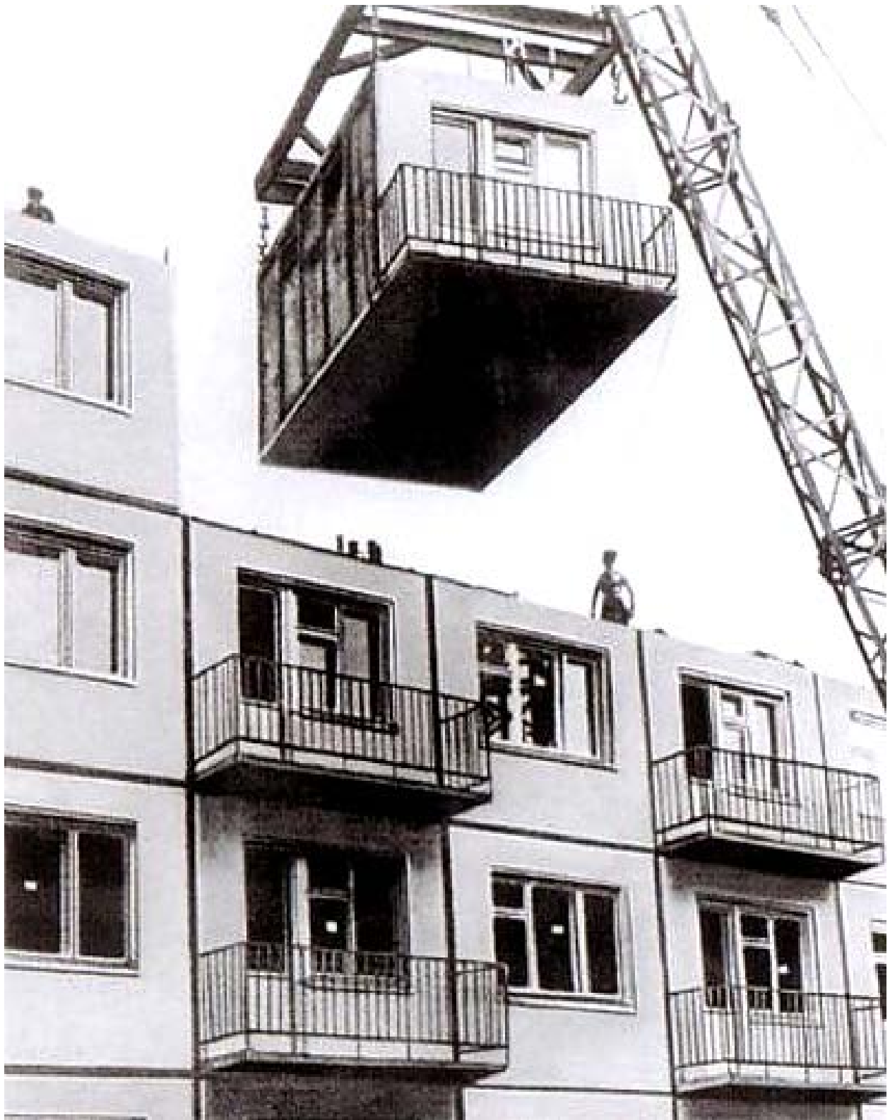
Crane assembly of a khrushchovka. Source: Photo Archives, Shchusev State Museum of Architecture. Moscow, 2019
