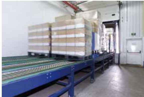
Source: Interlake Mecalux Automated Loading & Unloading System
