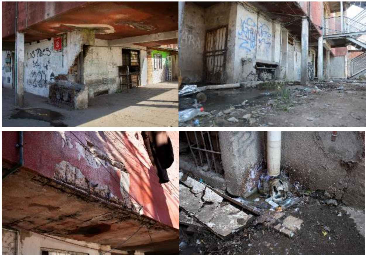
Figure 18. Building decay in the monoblocks
