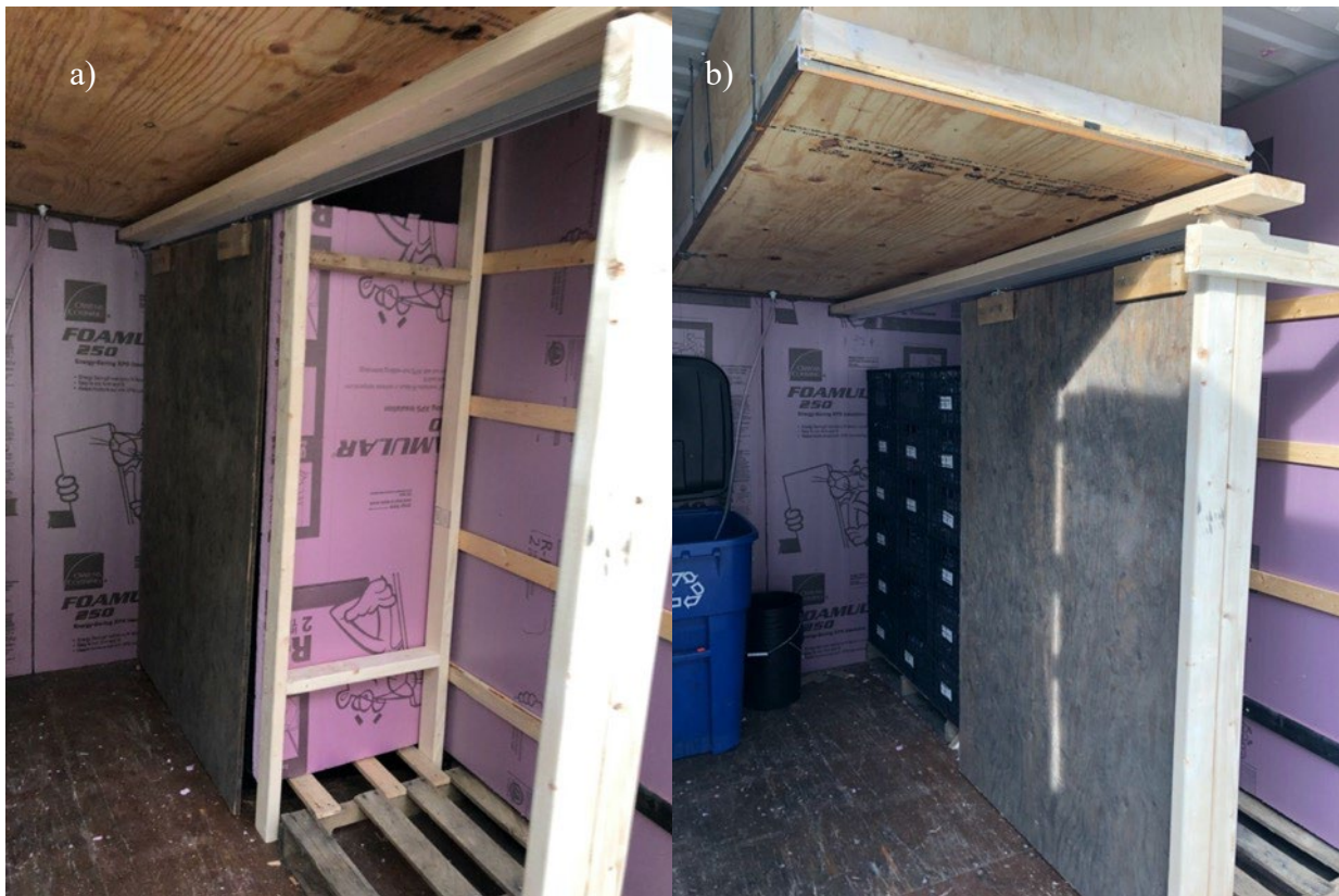
FIGURE A-5: Vegetable Crate Storage Compartment. a) vegetable crates insulated behind sliding door; b) vegetable crates seen with open sliding door.
