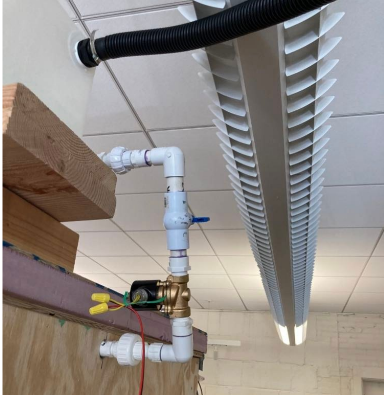
FIGURE 17: Assembled Plumbing Hardware. a) Top reservoir to cooling harness; b) full system.
