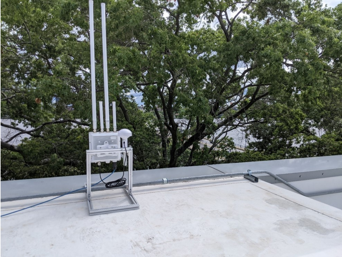
Figure 3-7: LoRa gateway installed on a rooftop
