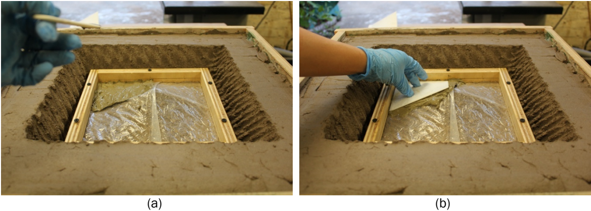
Figure 35: (a) Applying concrete to adobe formwork, and (b) measuring thickness of first layer
