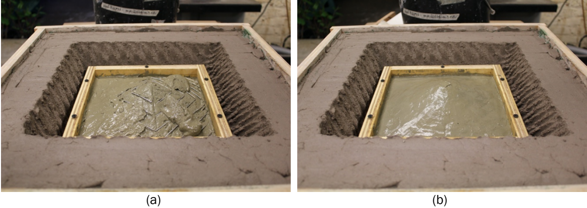
Figure 37: (a) Applying top layer of concrete, and (b) finished concrete shell on adobe formwork
