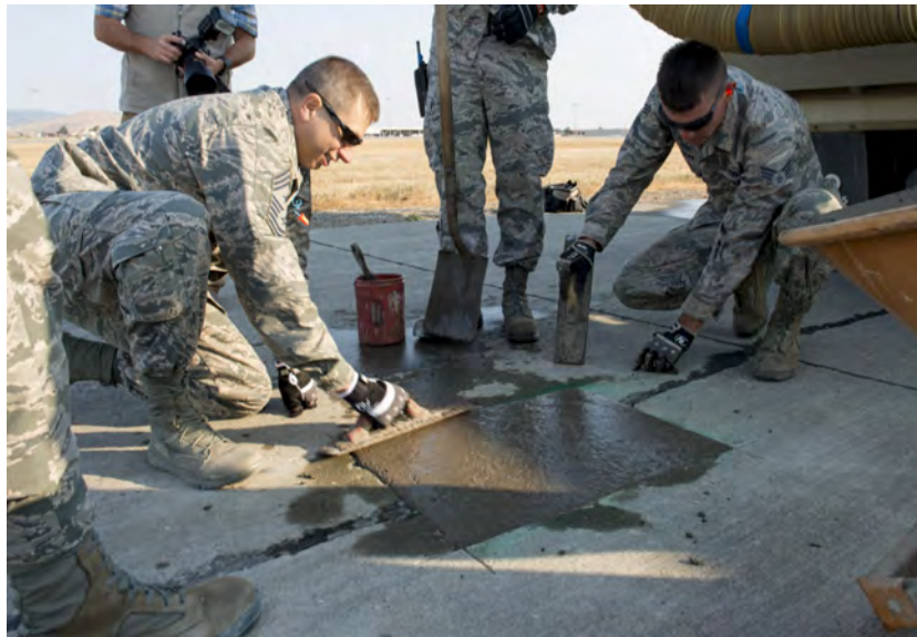
Figure 1-1: Air Force personnel work on repairing a section of runway. Image courtesy of: https://www.defense.gov/News/News-Stories/Article/Article/982954/air-force-engineers-repair-runway-in-iraq/
