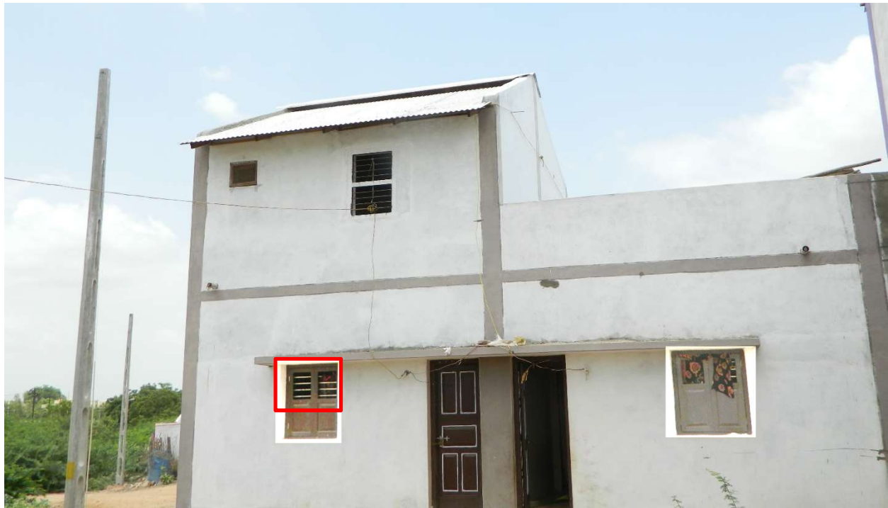
Figure 36: Rear view of the as-built Bhuj housing. Window areas have been color-enhanced to highlight open window area. Red box on left outlines the limited open area through the entire rough window opening. Similar open area on the right has been covered with cloth as a means to seal off the window.
