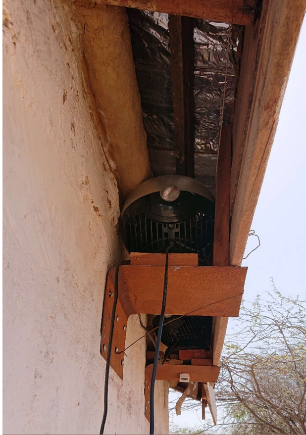
Figure 15: Fans Installed on Half of the Roof of the Structure (Bhuj, India)
