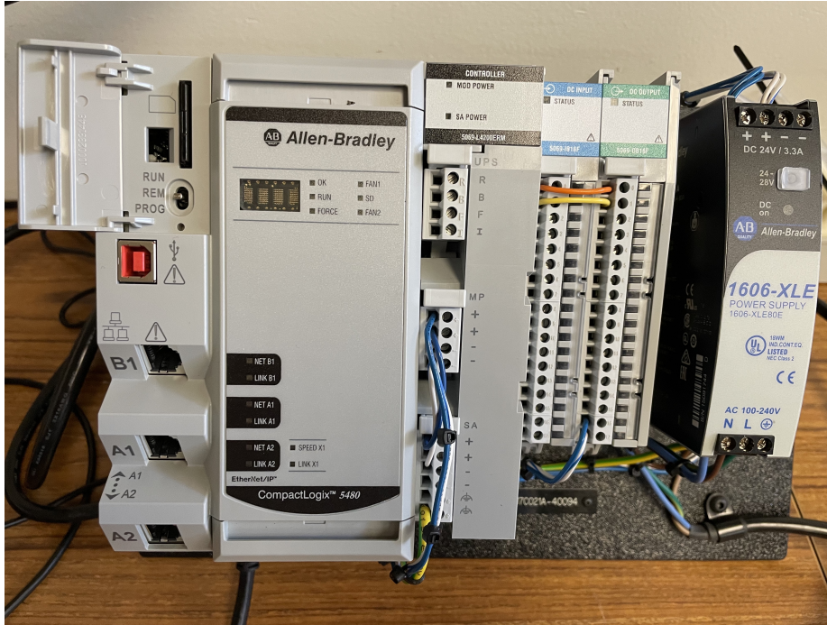
Figure 1-4: Allen-Bradley CompactLogix 5480 PLC in the DRL
