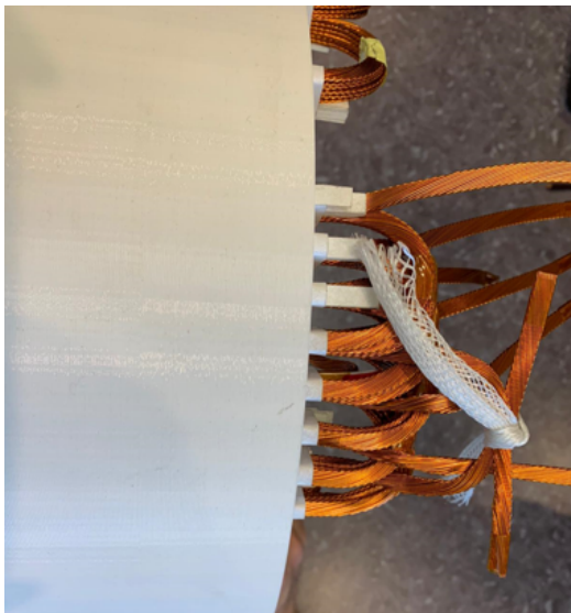
(a) Circular end turns from mockup test.
