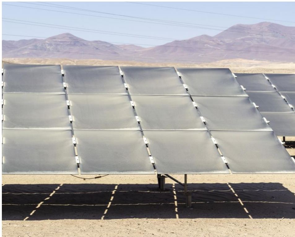
Figure 2-2. Dust accumulation on solar panels at Atacama solar park, Chile
