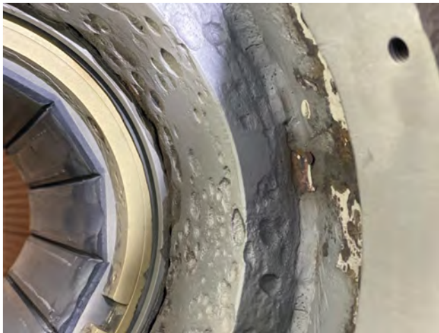
(a) Close-up view of sand blasted bearing housing.
