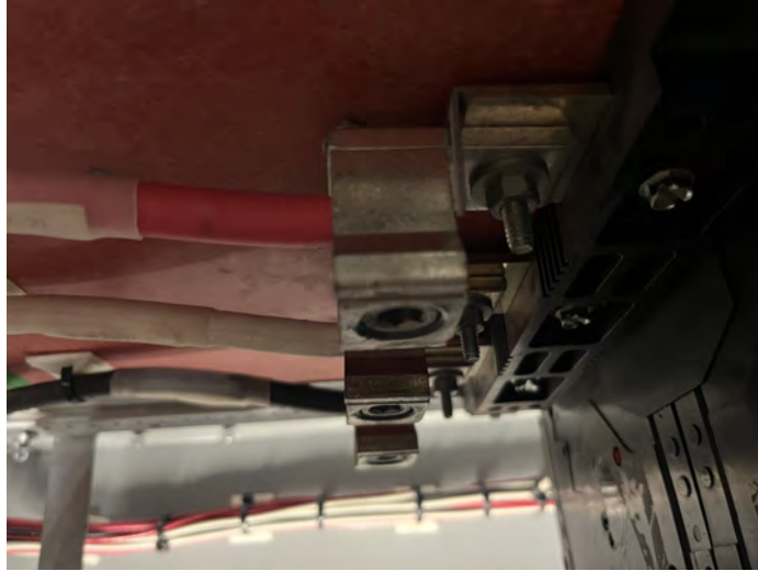
Figure A-21: USCGC WILLIAM CHADWICK (WPC 11050) Power Panel Interior
