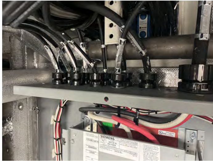
Figure A-17: Cable entries into the top of power panel 2DS-4P.
