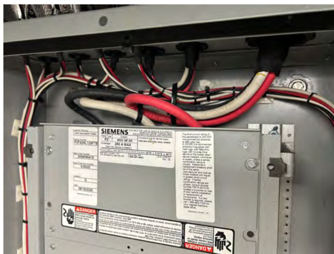
Figure A-20: USCGC WILLIAM CHADWICK (WPC 11050) Power Panel Interior
