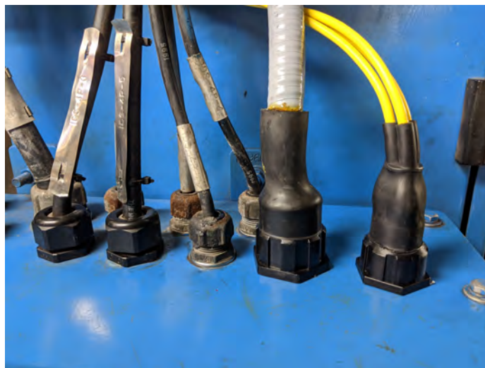
Figure A-16: Example of voltage leads (in conduit) and Conxall cables exiting from power panel.
