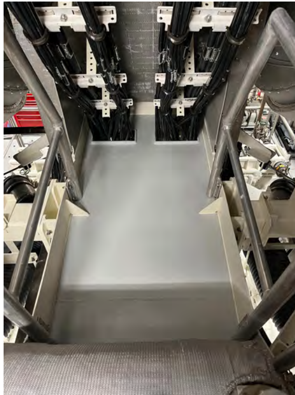
Figure A-7: Proposed installation location for AIO box on Engine Room 'Catwalk'
