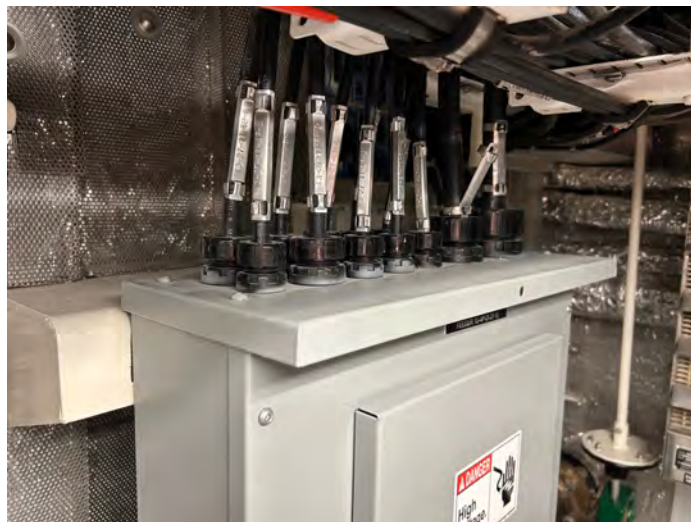
Figure A-18: Cable entries into the top of power panel 2DS-4P.
