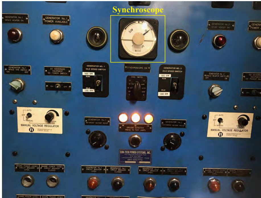
Figure 5-9: US Coast Guard cutter switchboard and synchroscope.
