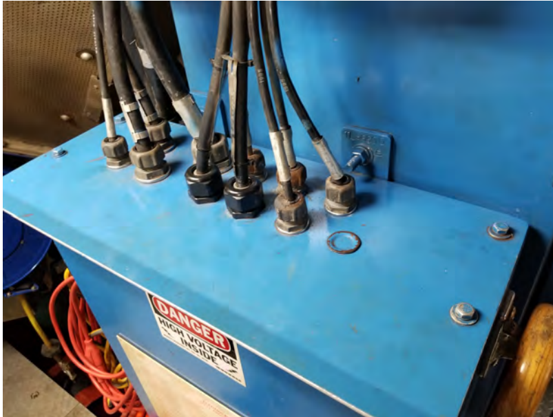
Figure B-9: Cable entries into the top of power panel 1DS-4P.
