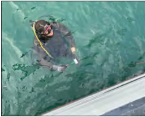
(a) Contracted Diver installing temporary reference electrodes in the water inside the stern tube covers.
