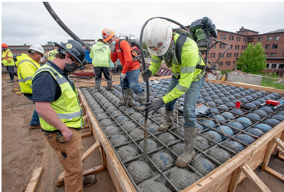
Figure 2-9: Casting of a concrete slab utilizing BubbleDeck technology for Western Michigan University
